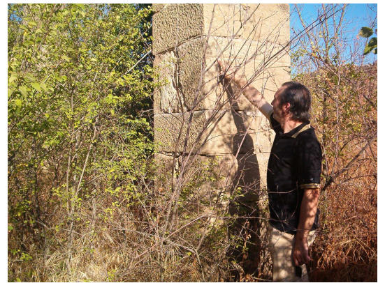
Fig. 2. Flood mark preserved in a column inside Serra's watermill remains at Mont-roig by the Sió River.
