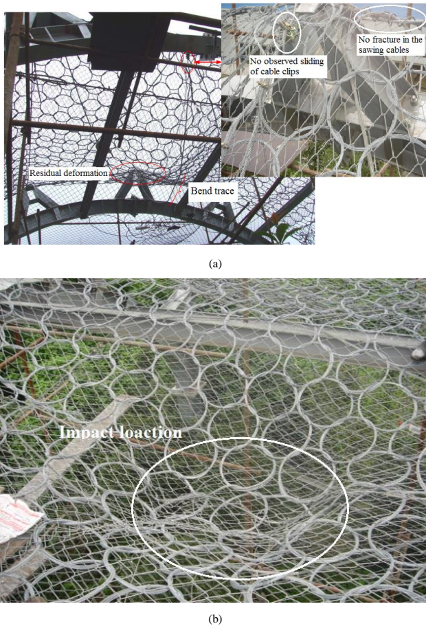
Fig. 10. The detail deformation of the components in the flexible rock-shed after the impact of the rock block.
